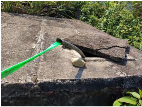
Water tank in Cooc village
